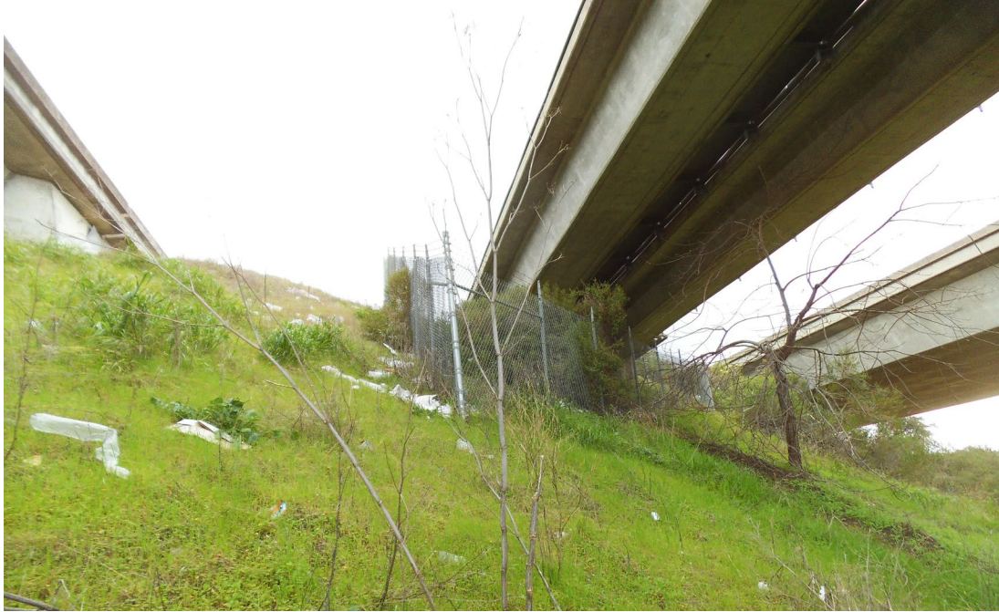
Note: Project site is the middle structure and the slope below, as viewed from Kinne Blvd., looking east. Figure 9. View of Concord Project Site C3015E
