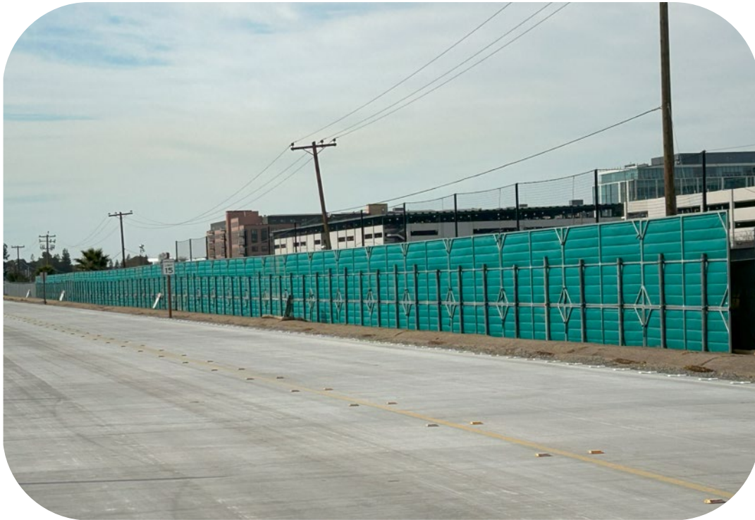
Installed courtesy screen for SJ Earthquakes Practice Field.
