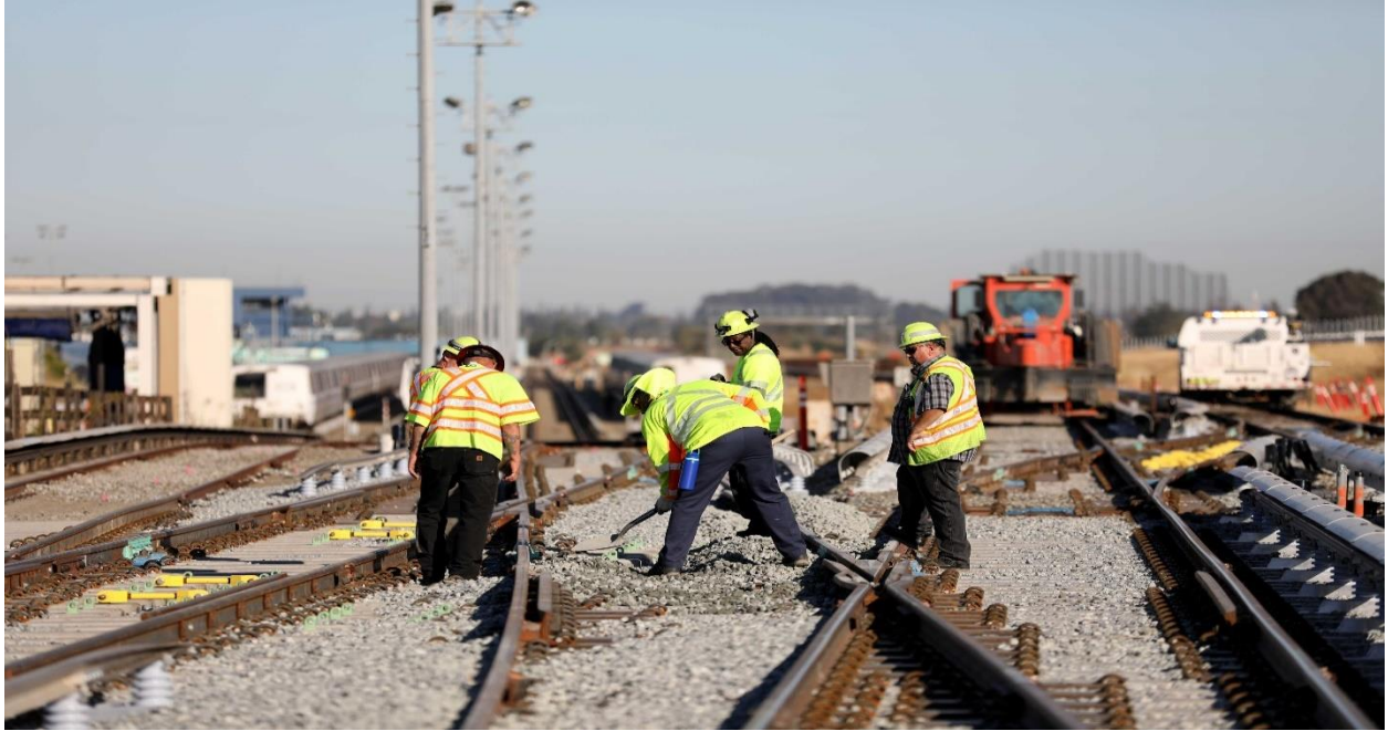
Description: Five employees in high visibility vests and helmets working on BART rail.
