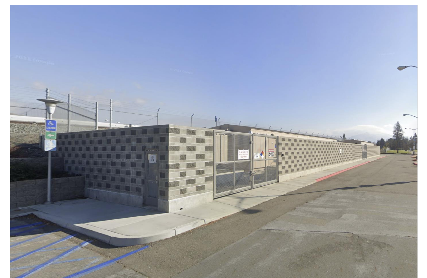
Example TPSS (Fremont Station)
