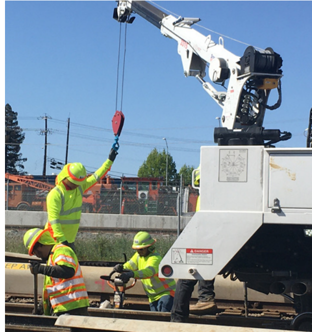
BART often utilizes cranes and forklifts to move oversized track components during weekend shutdowns.
