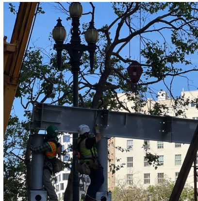
Tree Removal Tree Conflict with Entry Canopy
