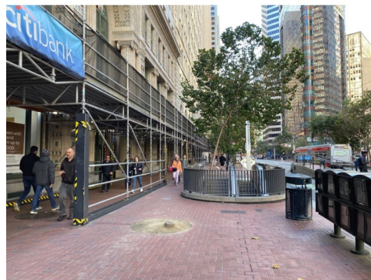
Coordination with Stakeholders Scaffolding Conflict with Entry Canopy
