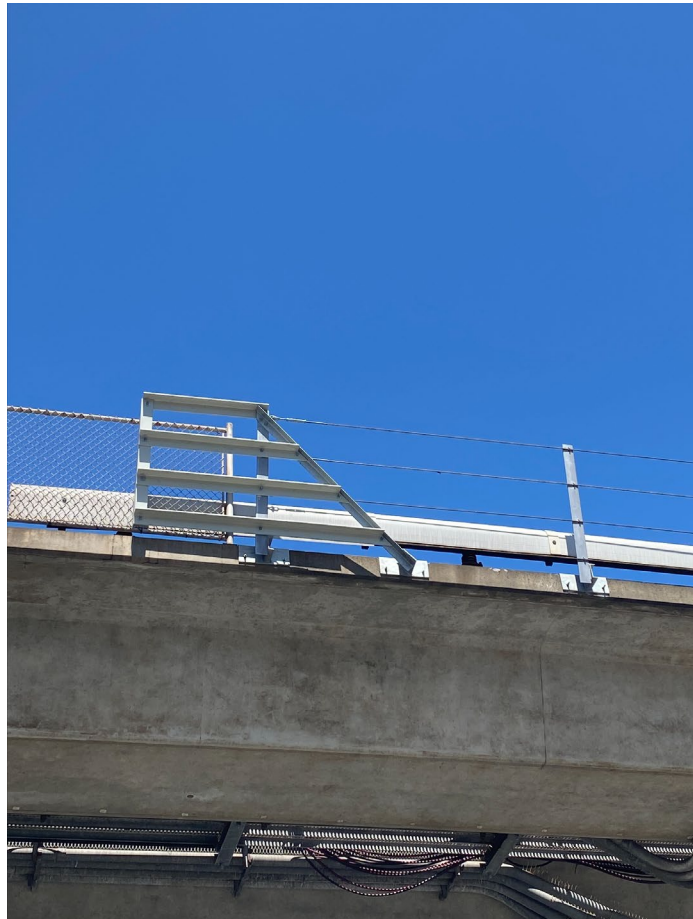
Completed A-Line Aerial Fall Protection at San Leandro BART Station (A40)
