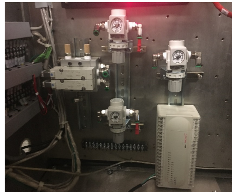
Solenoid /manifold block and pressure regulator used for the Cinch Mod
