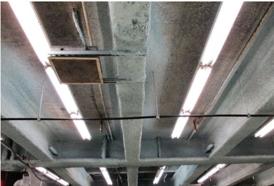
Measure RR will allow BART to renew and replace outdated mechanical infrastructure assets that are very important to safety – things like ventilation fans, fire service and suppression systems, and sewage pumps.
