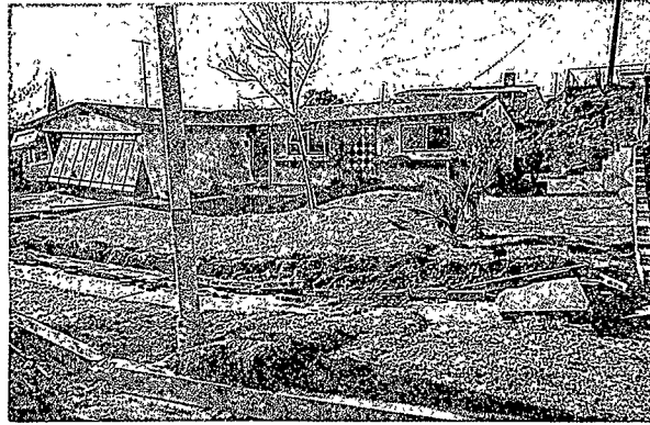
5-6 An example of structural damage caused by surface fault rupture.
