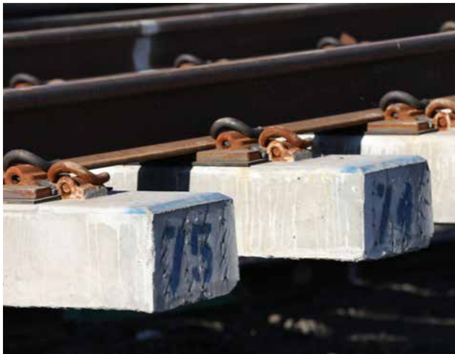
Cement ties like those to the right are replacing aging wooden ties and help to provide a more stable ride.
